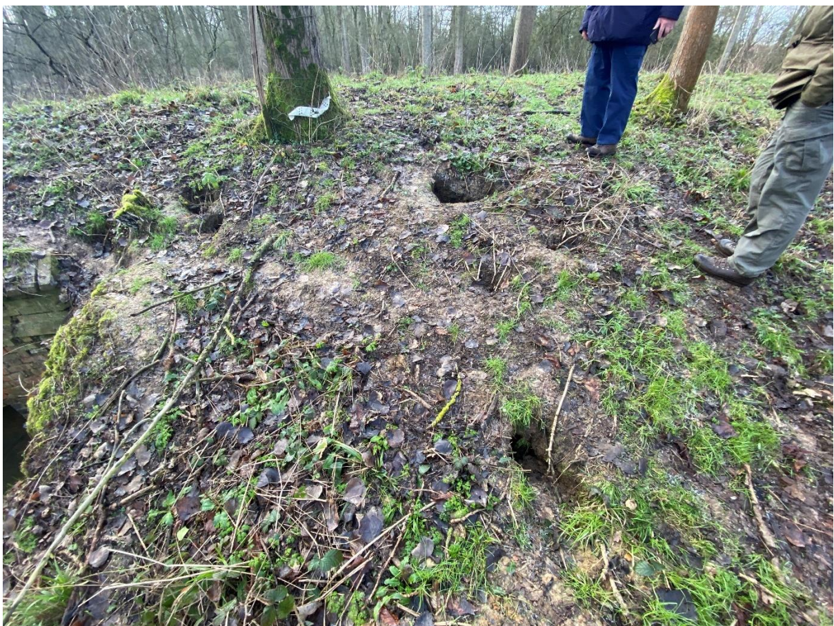
Plate 2 Example of badger burrows in the dam between the culverts.
